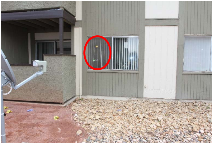
Exterior view of Apartment 156 and bullet hole
